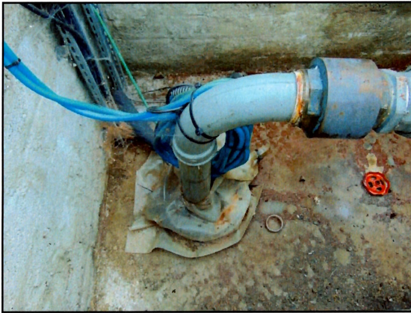
Photo 2 Ballycallan Muintir GWS borehole wellhead within chamber
