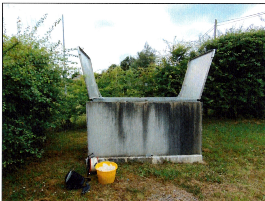
Photo 1 Ballycallan Muintir GWS borehole chamber
